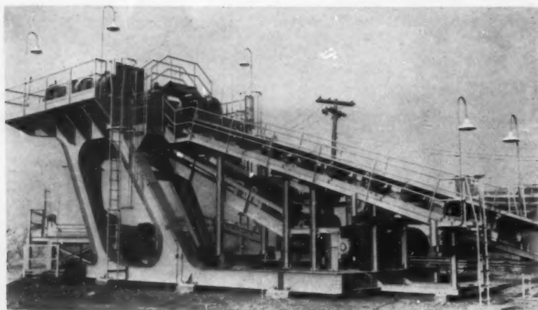
HEADFRAME at edge of pit contains drive machinery to power conveyor belt. Combination of three 200-horsepower motors gives belt speed of 600 feet a minute.
